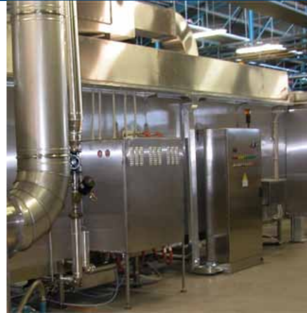
Tunnel system for mechanical components
